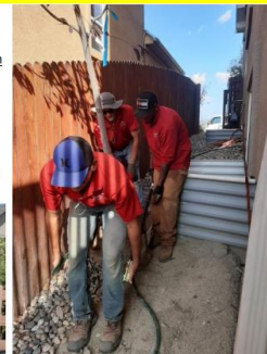
This site had very narrow access due to window wells. The trees had to be hand carried in. This site had additional charges.
